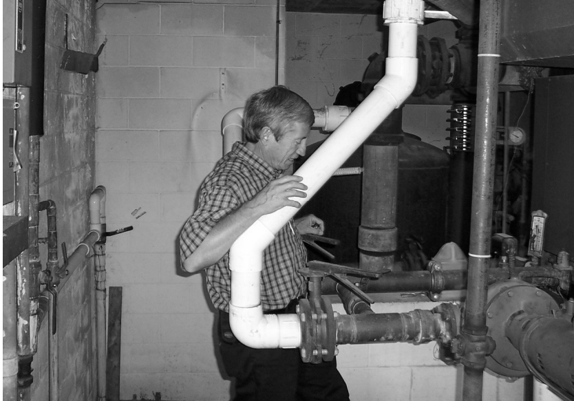
Park Superintendent Pat Mrsny is checking the pool heater in the mechanical room at Memorial Pool.
